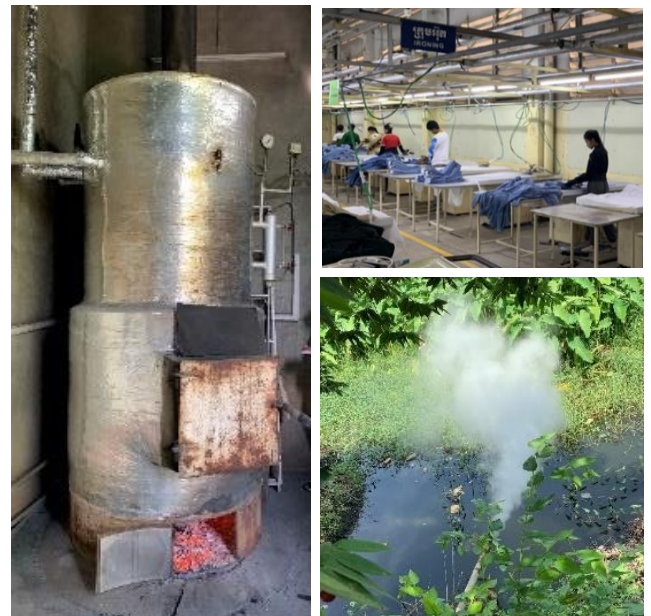
Figure 1: Boiler system before installation of condensate recovery
