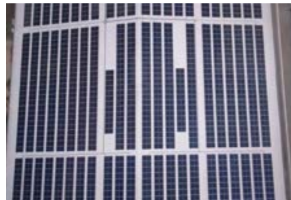
The eagle view of the PPSEC rooftop solar
